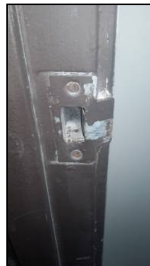
Rusted screw noted on groove plate
