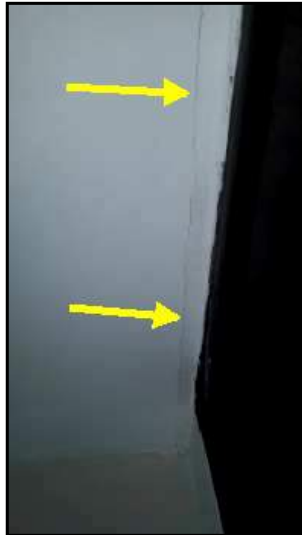
False ceiling board joints visible
