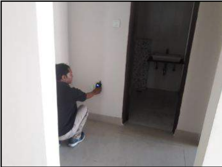
High moisture content on lower portion of front wall to the left side of bathroom 3 door
