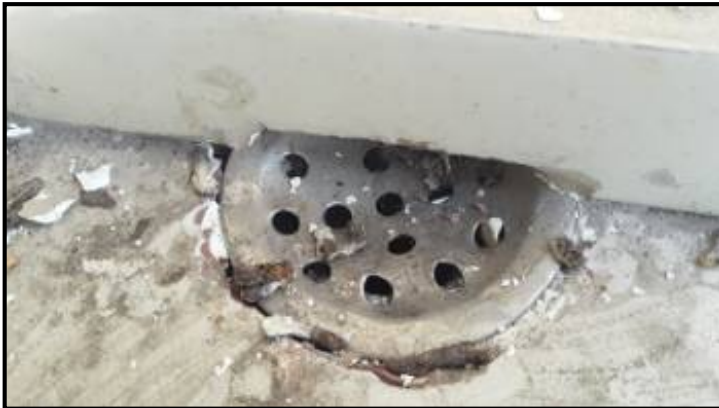
Grating partially under the wall and grouting not done
