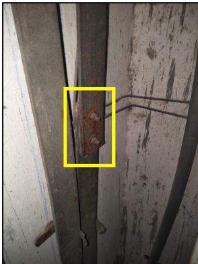
Welding not done at earthing plate joints
