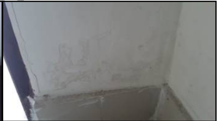
Moisture patches and paint deterioration noted on lower portion of left wall
