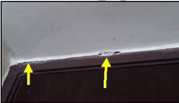
Gap noted at junction of false ceiling and head jamb of entrance door
