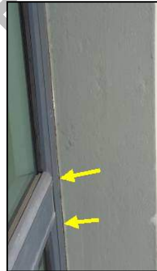
External gap noted around window frame
