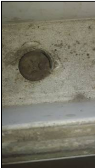
Rusted fastener on head jamb
