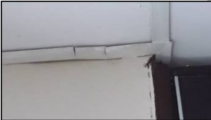
Damaged aluminium channel noted near front wall
