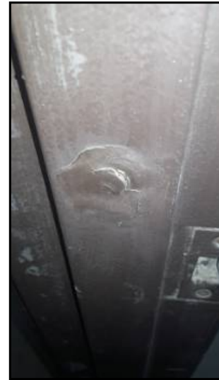
Fastener not concealed within door frame
