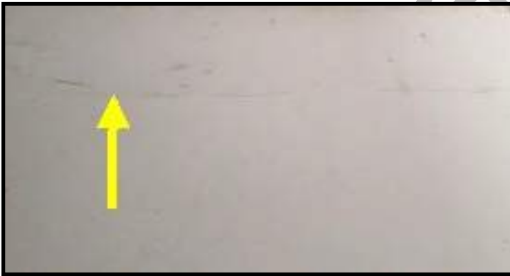
Crack noted on back wall upper portion
