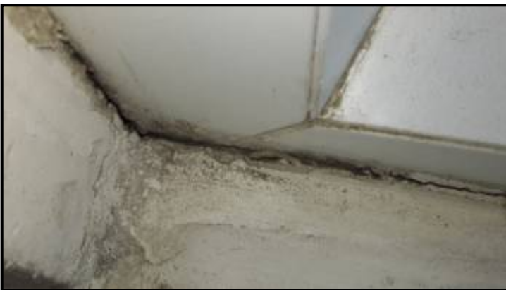
Gap noted at junction of window frame and wall on inside
