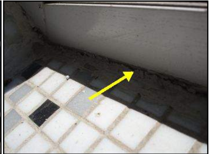
Non uniform putty filling noted at junction of window frame and wall tiles
