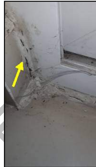
Sealant deterioration at junction of balcony door and skirting
