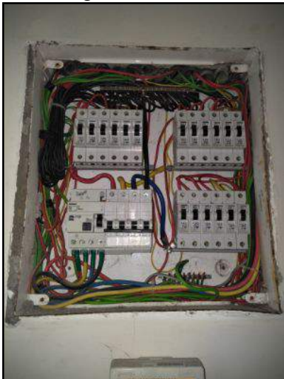
Wire dressing not done properly inside DB
