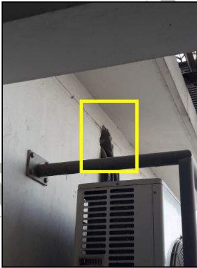
Packing not done on external wall around AC pipe sleeve
