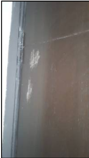
Paint deterioration noted on panel laminate
