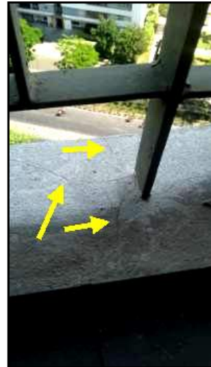
Multiple cracks noted on railing sill
