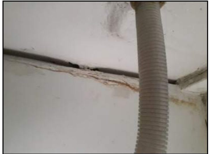
Sink counter cabinet : Rear side head plank is damaged due to water infiltration
