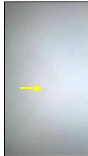
Hairline diagonal crack noted on back wall at mid height to the right side of junction with column
