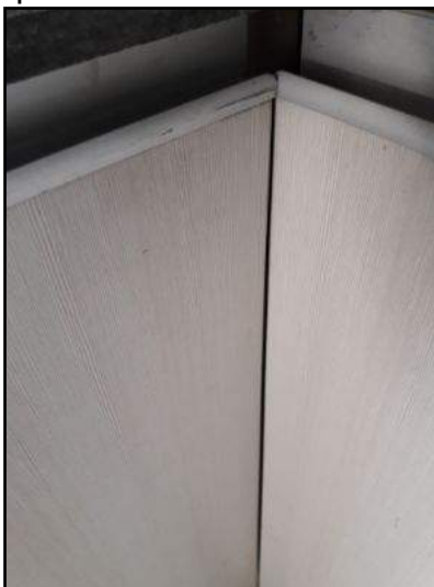
Right side counter cabinet : Last panel is not opening
