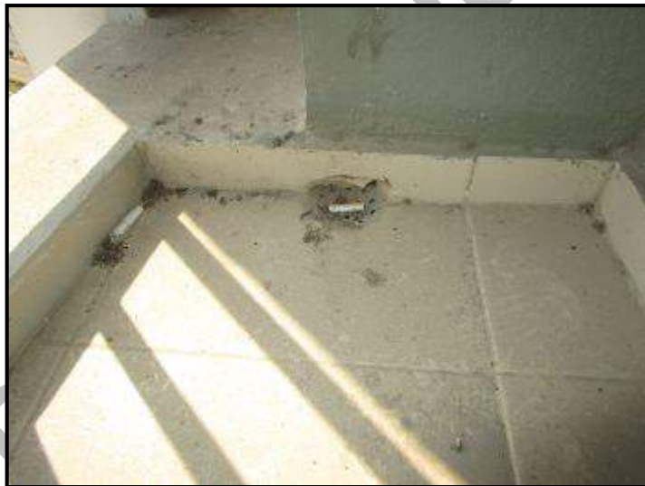
Right side grating near bedroom 3 is partially under the wall
