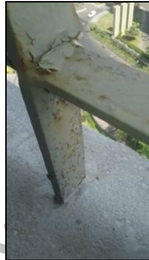
Paint peeling off and rust noted on MS rail
