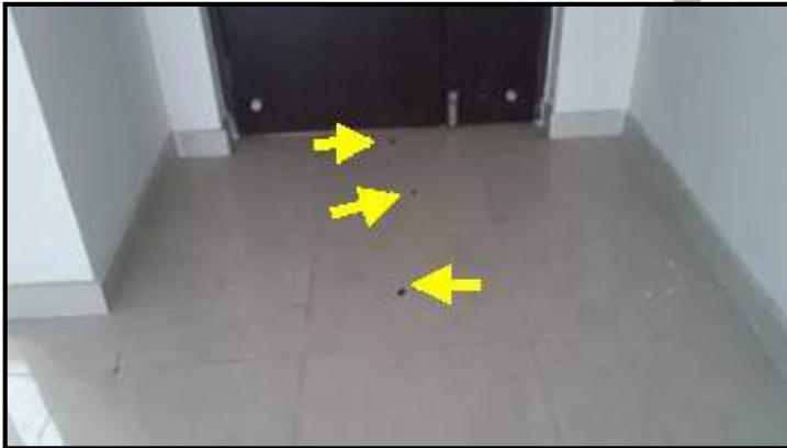
In front of entrance door : All tile except the marked ones are hollow
