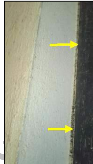
External gap noted around window
