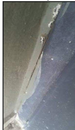
External gap noted between balcony door frame and wall
