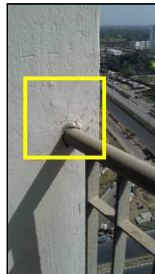
Crack and hollow plaster noted around ms rail fixation with wall
