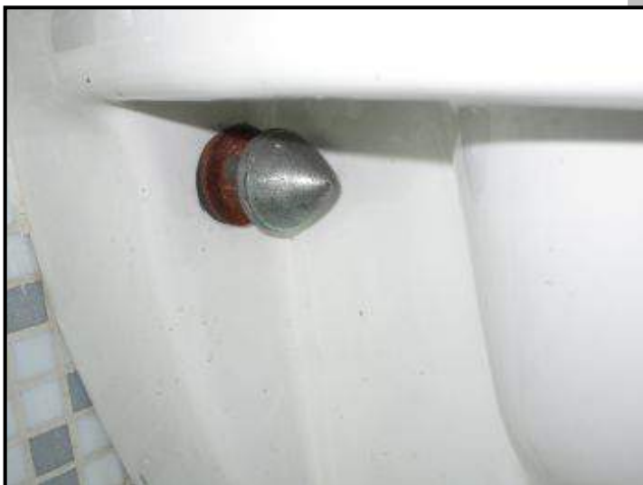
Rusted washer noted on WC
