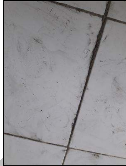
Inadequate tile joint filling noted at places
