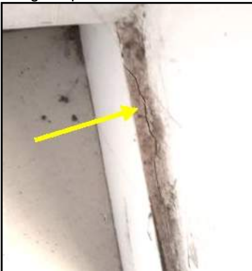
Detachment of skirting from left wall noted near balcony door
