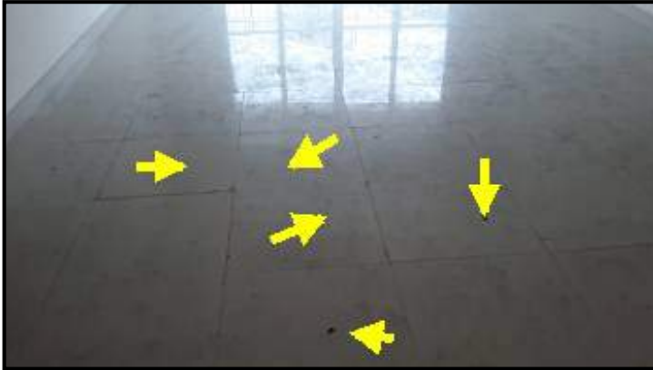
In middle and near front wall : All tiles except the marked one are hollow
