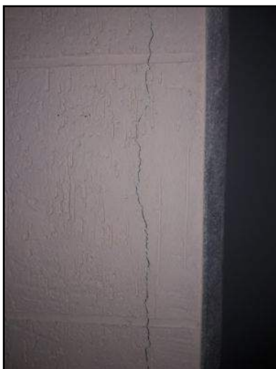
Crack noted on back wall near lift
