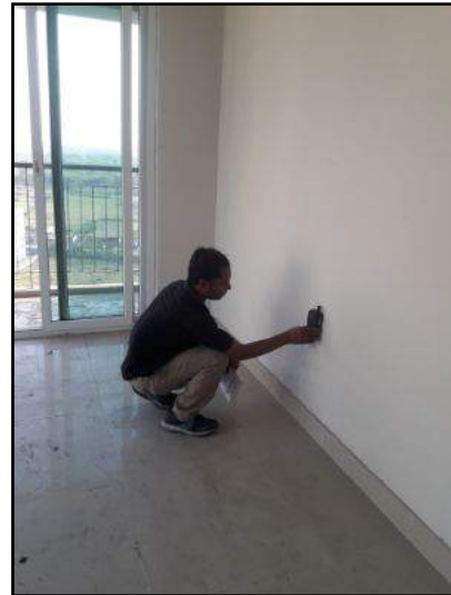
High moisture content on lower portion of right wall below AC
