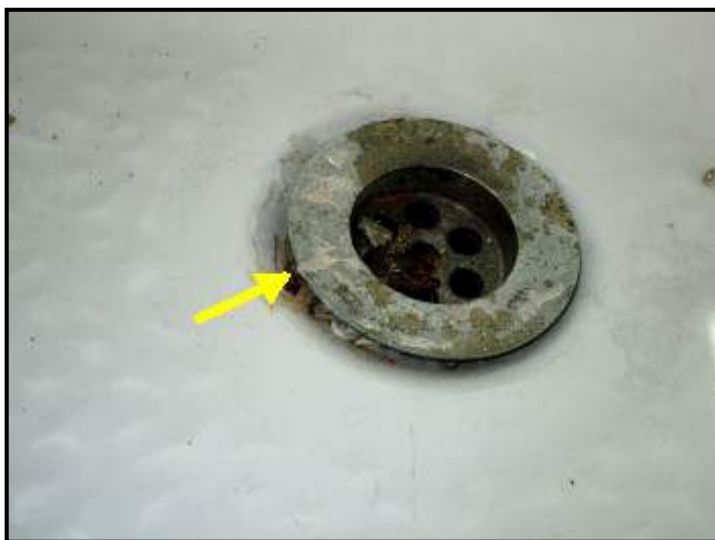
Gap noted around bathtub waste
