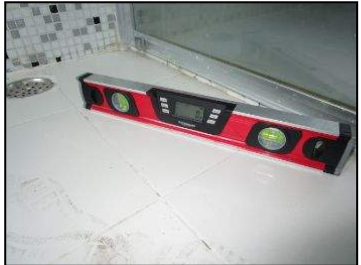
Water pockets noted in shower area around near shower area sliding door
