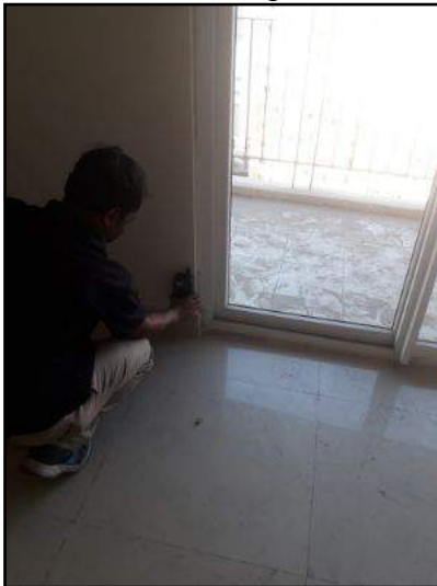
High moisture content on front wall to the left side of balcony door
