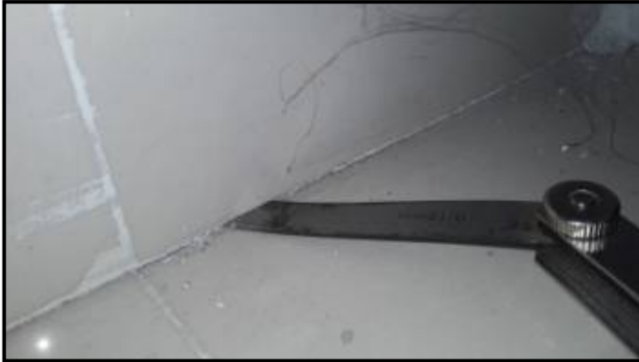
Gap noted at junction of right wall skirting and floor tile near entrance door
