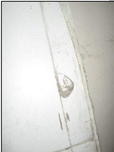
Damaged floor tile noted near entrance
