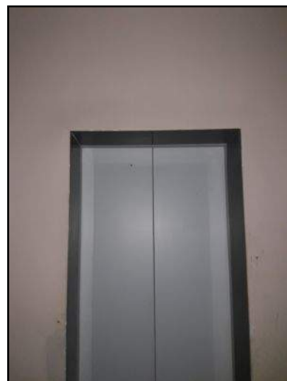
Signage not provided for service lift
