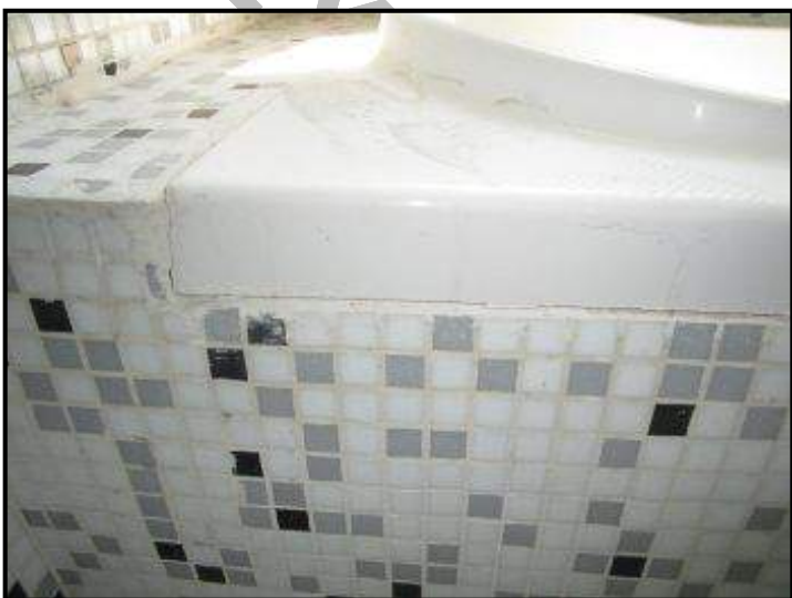
Gap between bathtub and walls around
