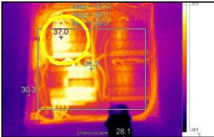
Infrared image showing hot MCB at the DB
