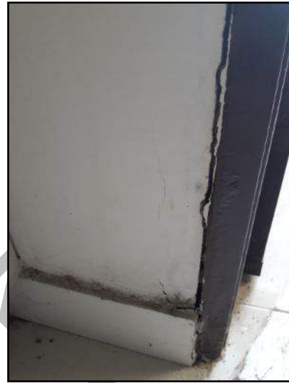
Distinct crack along the wall and door frame
