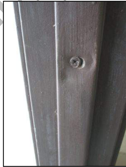
Fasteners visible on door frame
