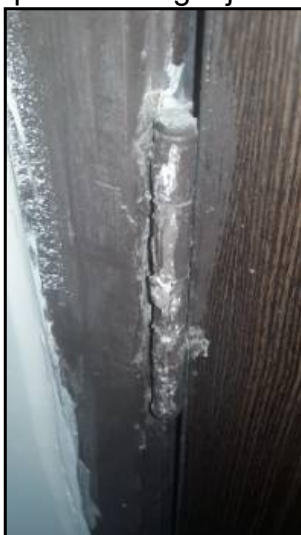
Paint deterioration noted on door hinge
