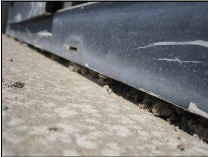
External gap around window frame
