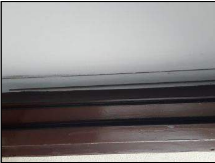
Gap between false ceiling and wall surface above kitchen balcony door frame
