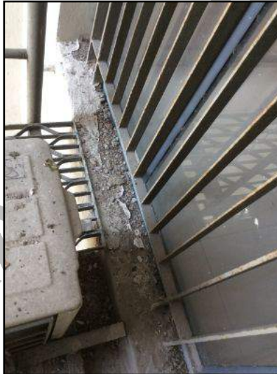
Broken plaster noted on exterior sill of window near entrance door
