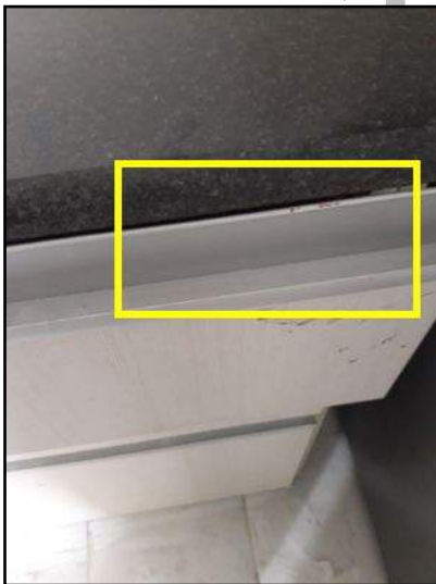
Top drawer aluminium channel operating handle is flashing with counter top
