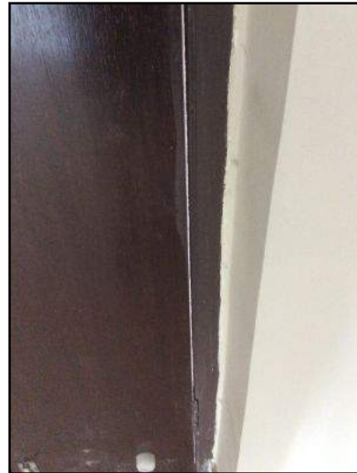
Gap between smaller panel and frame on closing
