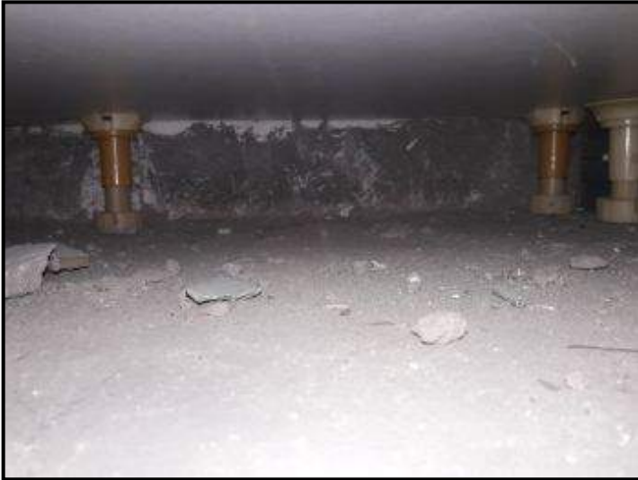
Skirting not provided behind the cabinet
