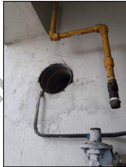
Cowl not provided at vent terminal
