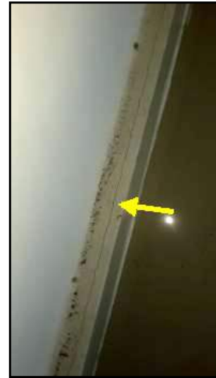
Crack noted at junction of back wall and skirting
