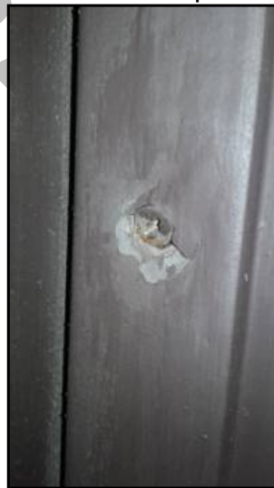
Fastener holes not filled
