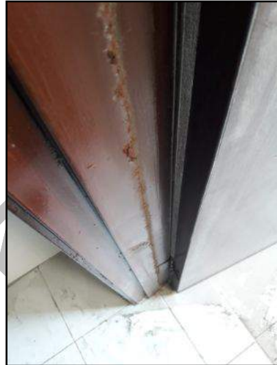
Rust noted on door frame
