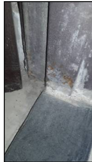
Surface rust noted on door frame
