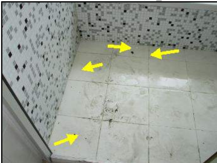
4 nos hollow tiles noted in shower area
