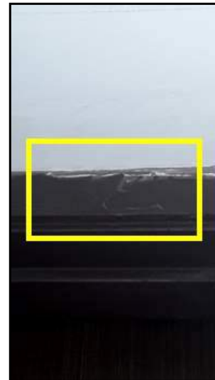
Paint peeling off noted on head jamb
