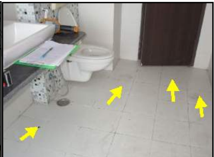
4 nos hollow tiles noted in WC area
