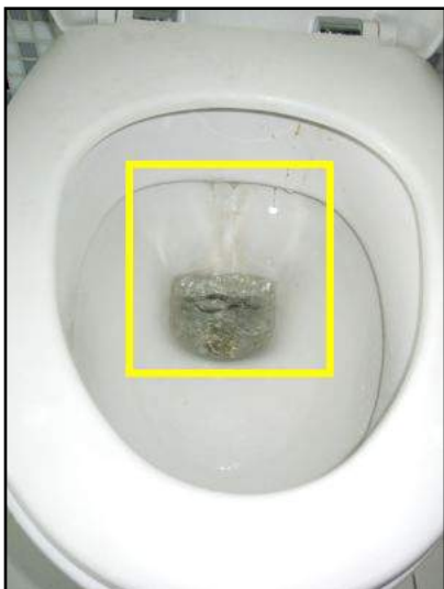
Continuous flow of water at the WC
