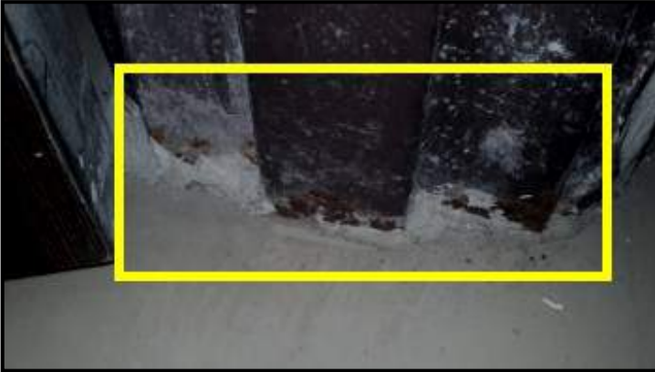
Surface rust noted on lower portion of right jamb
