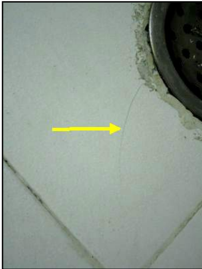
Crack on floor tile near shower area grating
