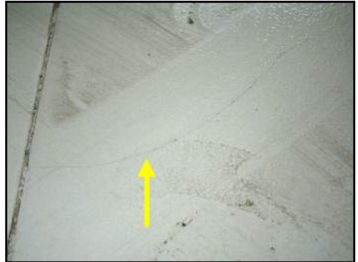
Crack noted on floor tile at middle portion near basin counter
