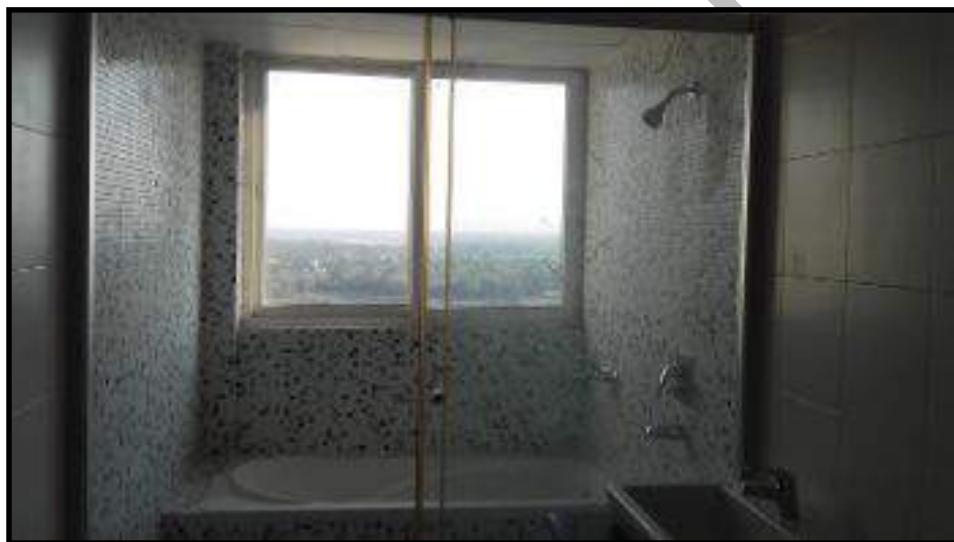
Provision for exhaust not provided
