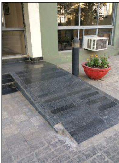
Hand rail not provided at ramp
