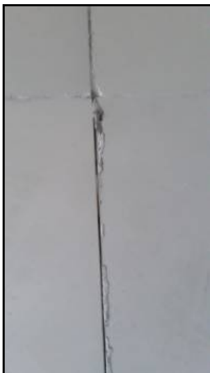
Joint filling not done on floor tile joints near right side corner of front wall
