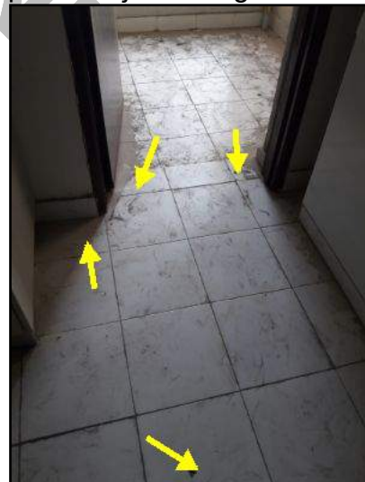
4 hollow tiles noted near balcony door
