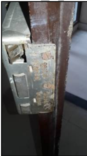
Rusted screws noted on lock
