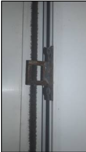
Surface rust noted on lock keeper plate
