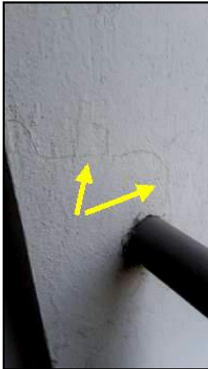
Significant diagonal crack noted on left wall near bedroom 4
