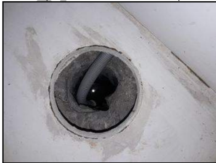
Grating not provided at outlet
