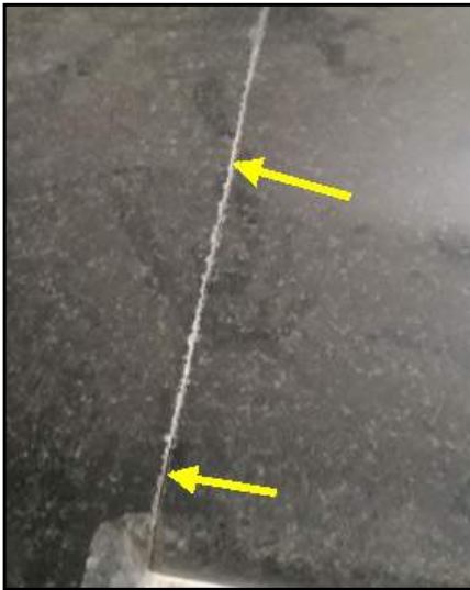
Inadequate joint filling noted on counter top
