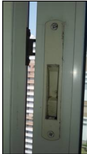
Left side panel lock not working
