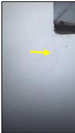
Hairline diagonal crack noted on back wall under left side reveal of window
