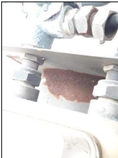
LPG meter plate rusted
