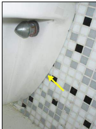
Gap between WC and wall
