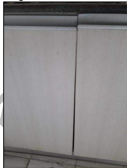
Panels are misaligned for right side first cabinet near fridge
