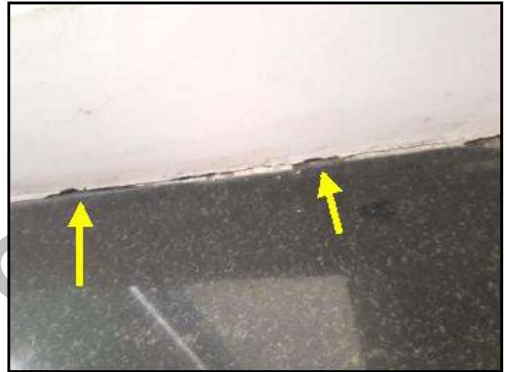
Left side counter top loosely fitted and distinct gap with wall
