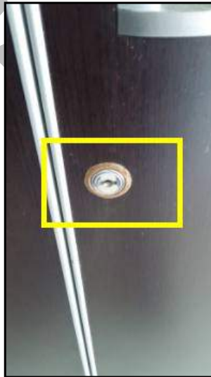
Surface rust noted on lock hardware of cupboards
