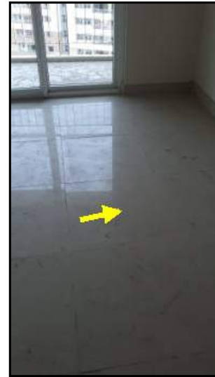
Near front wall right side corner : All tiles except the marked one are hollow
