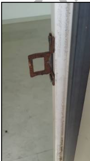
The keeper is protruding out of the door edge
