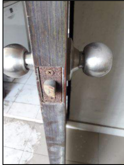
Rusted lock plate
