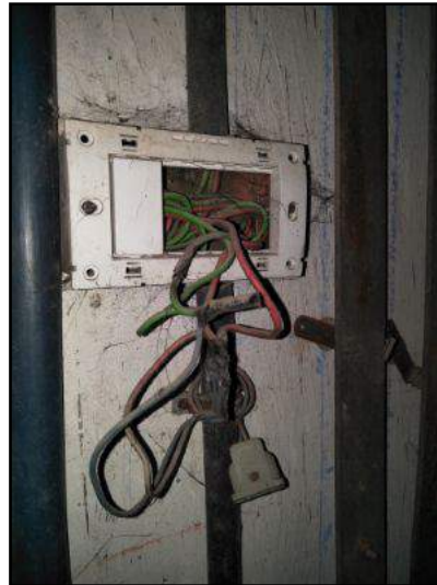
Switch and socket not installed in socket board
