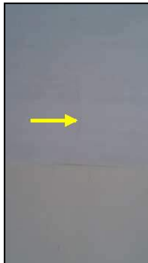
Crack noted on plaster ceiling near left wall above right reveal of left alley opening
