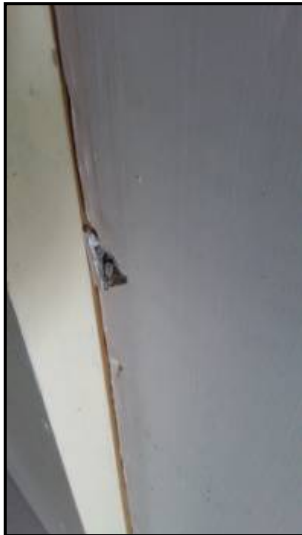
Broken false ceiling board noted near entrance
