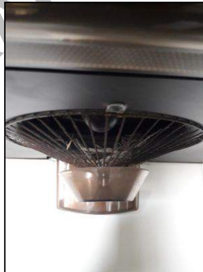
Exhaust grill rusted
