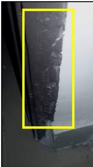
Uneven surface finish noted on inside lower portion of right jamb
