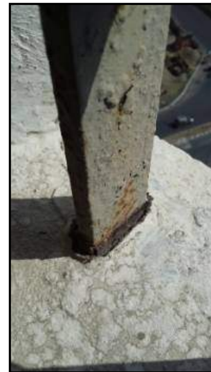
Surface rust noted on MS rail
