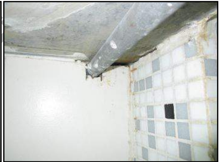
Gap noted around counter support
