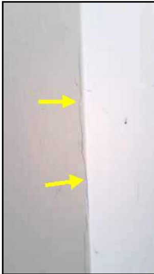
Significant vertical crack noted on front wall corner with right wall
