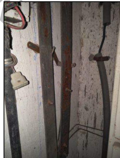
Rust noted on earthing plates
