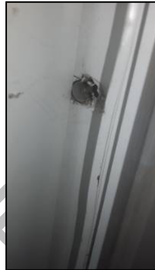
Fastener screw cap not installed
