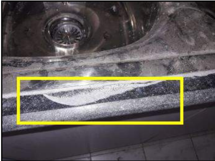
Grinding not done on counter top near sink
