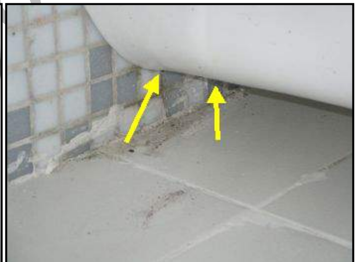
Visible patches at WC bottom due to leakage
