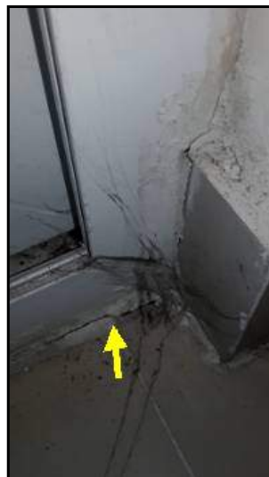
Sealant separation noted at junction of floor tile and balcony door
