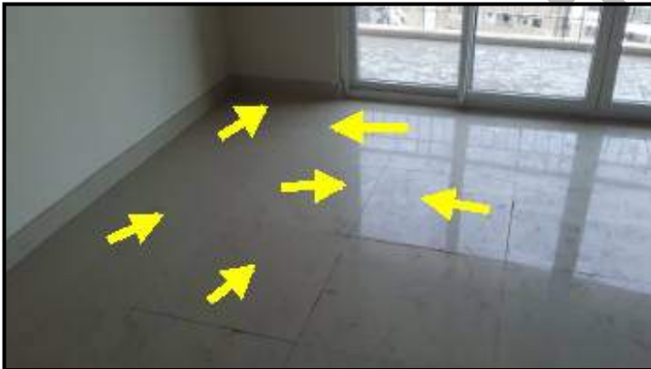
Front wall left corner : Marked tiles are loosely fitted
