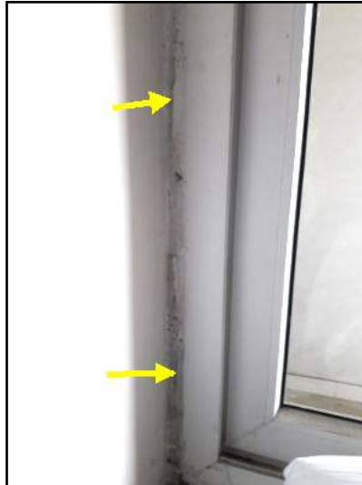
Inadequate application of filler
