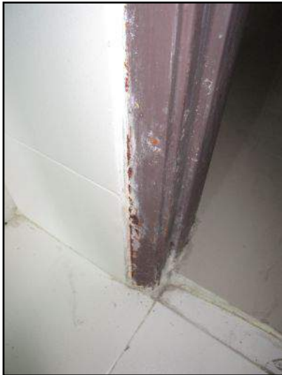
Surface rust noted on door frame
