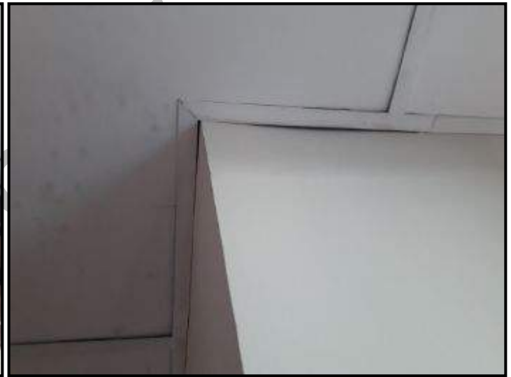
Uneven gap noted at junction of false ceiling and wall surface
