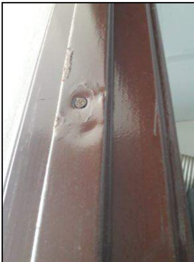
Fasteners not concealed within frame
