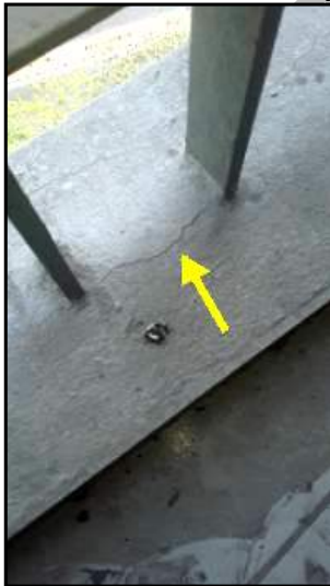
Crack noted on railing sill opposite to bedroom 3
