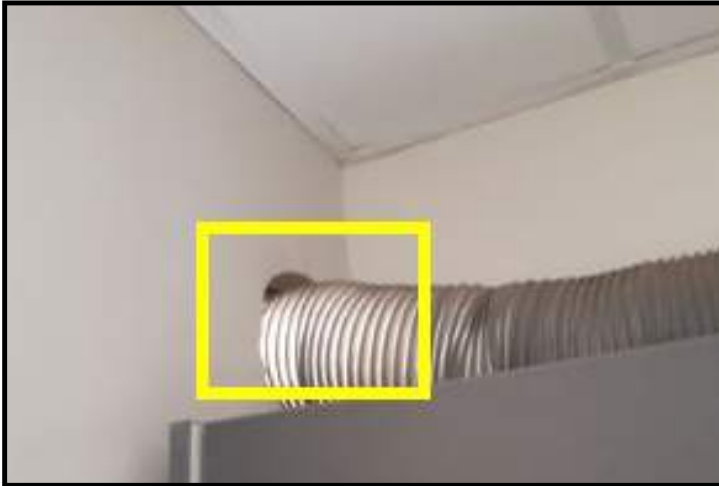
Gap around chimney vent sleeve
