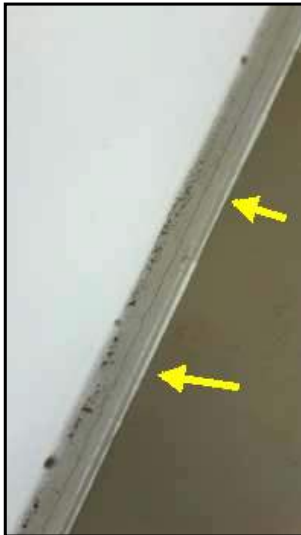
Hollow back wall skirting noted near corner with left wall
