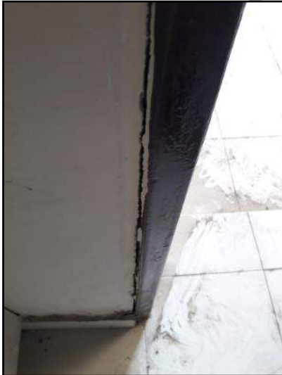
Unstable door frame due to crack at junction of left jamb and wall
