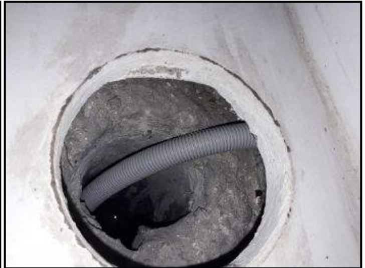
Cement heap noted around floor drain outlet
