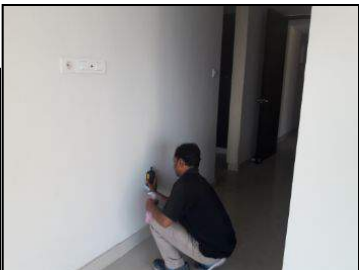
High moisture content on right wall lower portion near switch board
