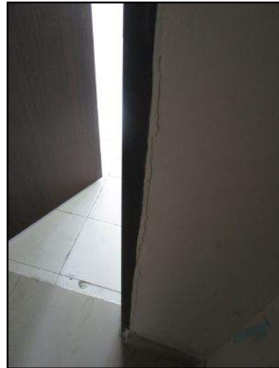
Crack running along the frame and wall
