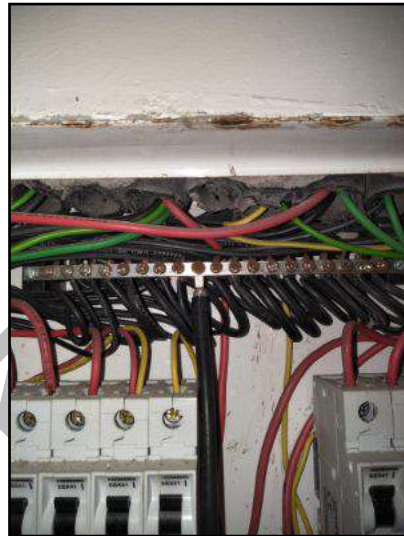
Neutral bar screws rusted
