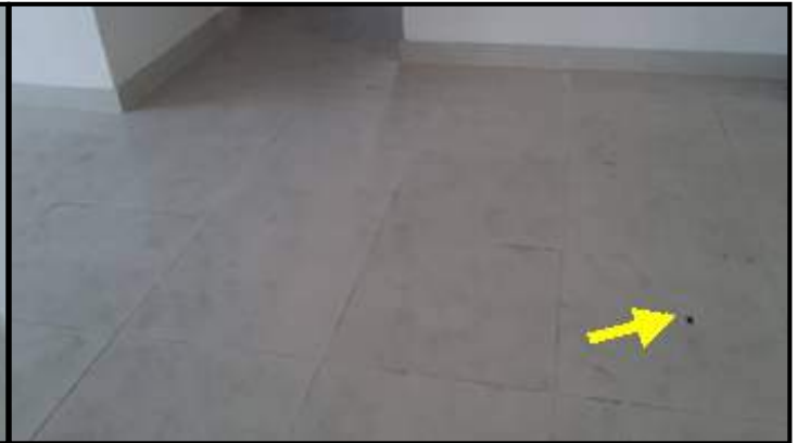
Near right wall : All tiles except the marked one are hollow
