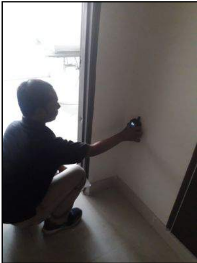
High moisture content on front wall
